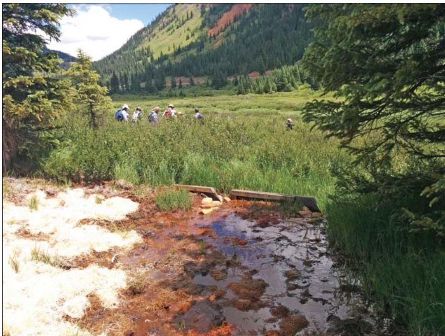
NPSNM members behind a ditch plug structure at Chattanooga fen. Photo: Dana Price
